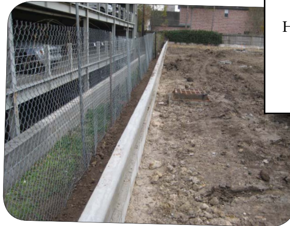
The retaining wall along the east property line has been completed and is ready for backfill.
