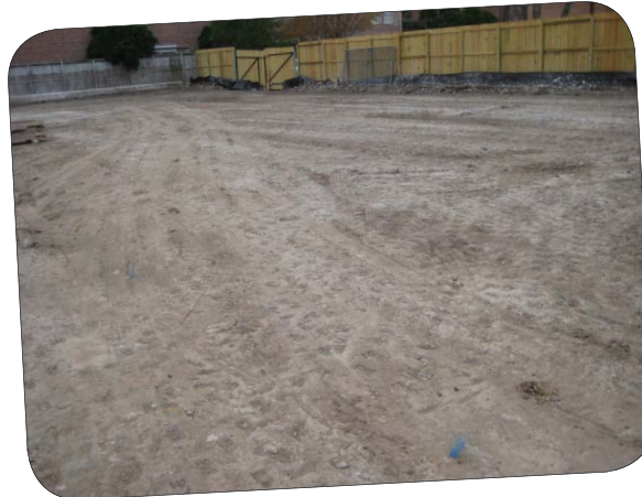
Pictured above is the southwest parking lot; it is ready for the asphalt paving base.
