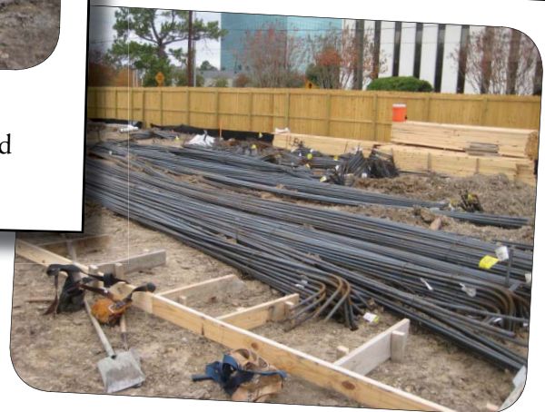
The rebar has been delivered. It will be used for building grade beam foundations.
