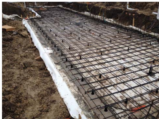
Pictured above, the rebar and waterproofing is in place for the seminar room slab of The Hope and Healing Center .
