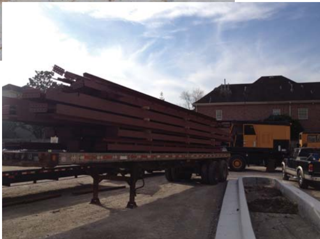
Below left, the first load of steel onsite is ready to be unloaded.
