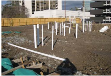
Underground plumbing installed for kitchen area in The Youth/Young Adult and Scout Facility.
