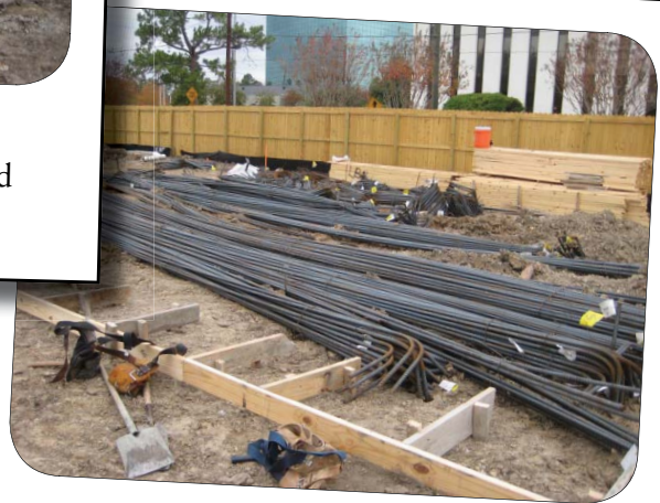
The rebar has been delivered. It will be used for building grade beam foundations.
