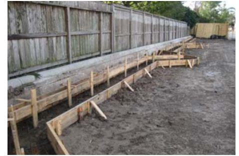
Curb and gutter formwork at west parking lot ready to receive concrete.
