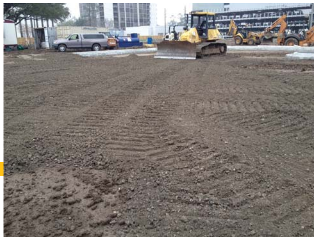
Pictured at right, the crushed concrete base is being installed at the southwest parking lot.
