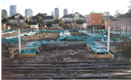
Preparation for the main entrance to the The Youth/Young Adult and Scout Facility.
